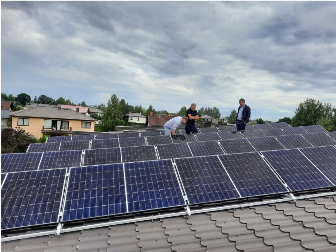
Figure 11. Rooftop solar facilities at the row houses building
