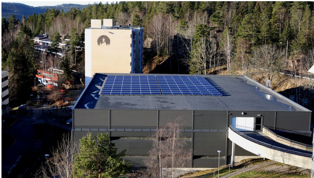
Figure 1. Rooftop PV at Røverkollen housing cooperative
